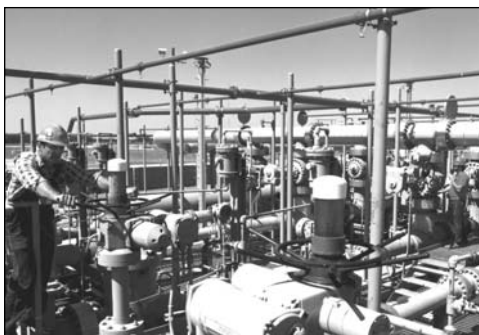
Employees work on piping at the Strategic Petroleum Reserve in West Hackberry, Louisiana
