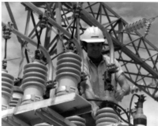
Southwestern Power Administration's Poplar Bluff, Missouri, switchyard.
