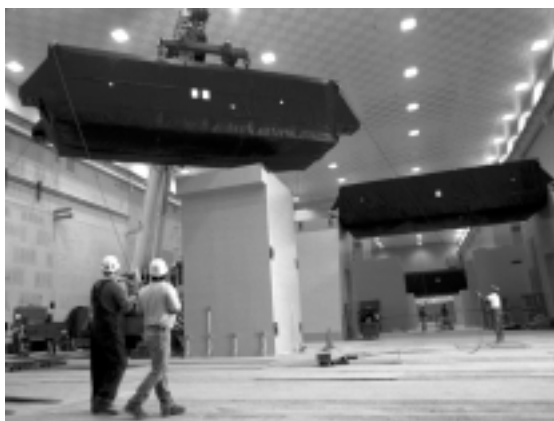
Installation of NIF Spatial Filter End Vessels in Laser Bay 2 at Lawrence Livermore National Laboratory.
