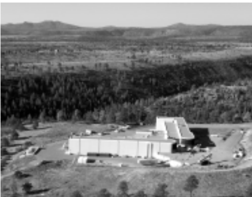
The following photograph shows DARHT's main facility, the Hydrotest Firing Site, under construction.
