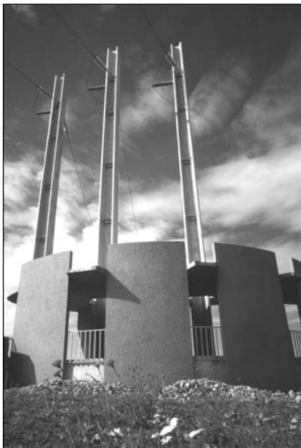
Bonneville Power Administration's beautified special transmission structure near Hood River, Oregon
