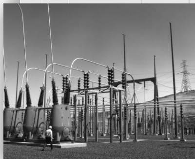
Equipment yard at Bonneville Power Administration's Celilo Converter Station
