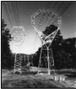
Six-Phase Electric Transmission Tower
