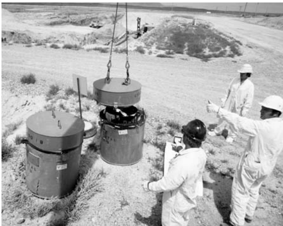
Waste Receiving and Processing at Hanford Site.
