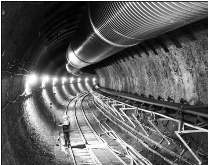
View of an exploratory tunnel at Yucca Mountain dug by a 25-foot-diameter tunnel boring machine.
