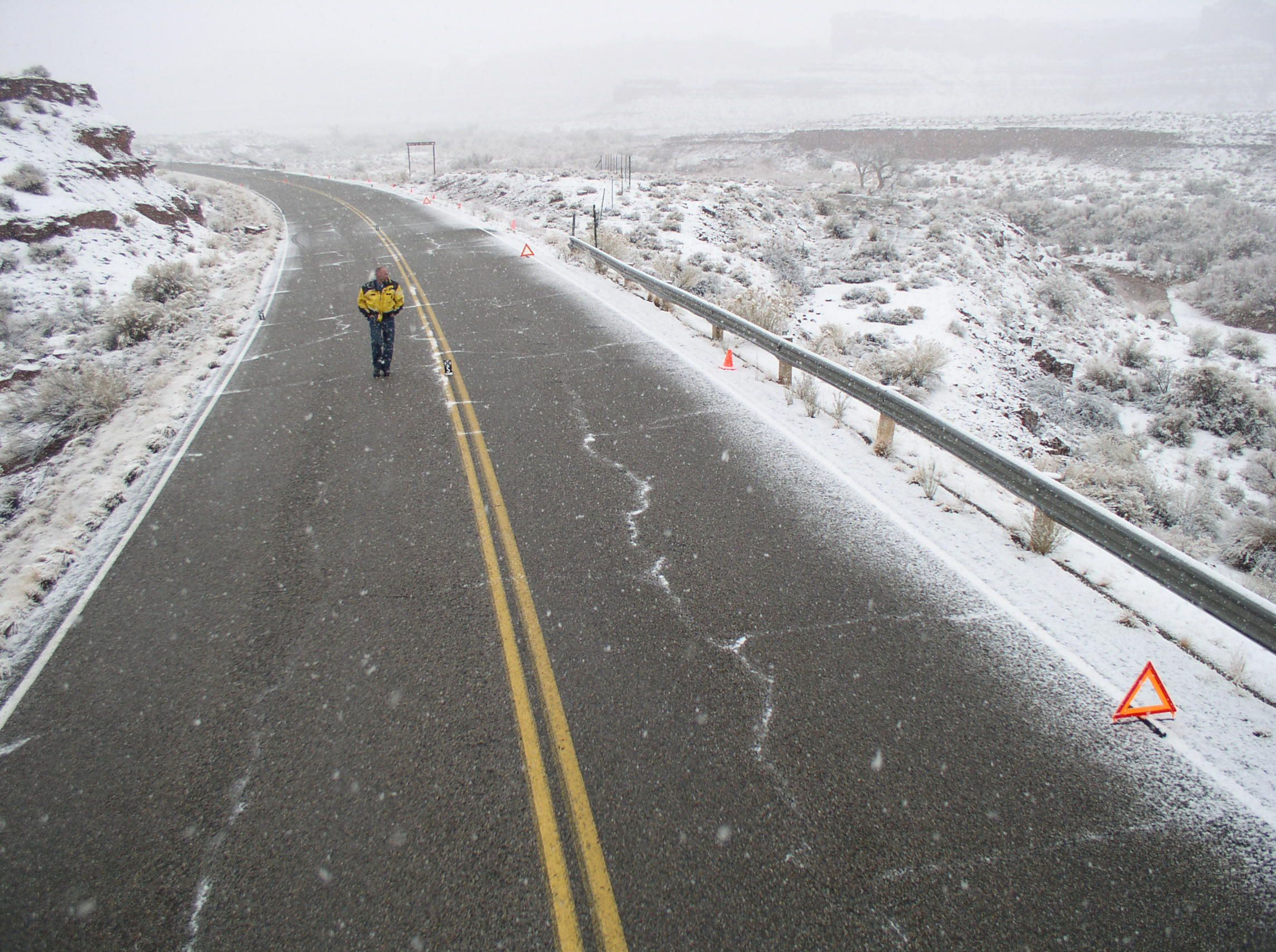
Hwy. Photo #40 - View of guardrail, curve, and first embankment that had a 2:1 slope
