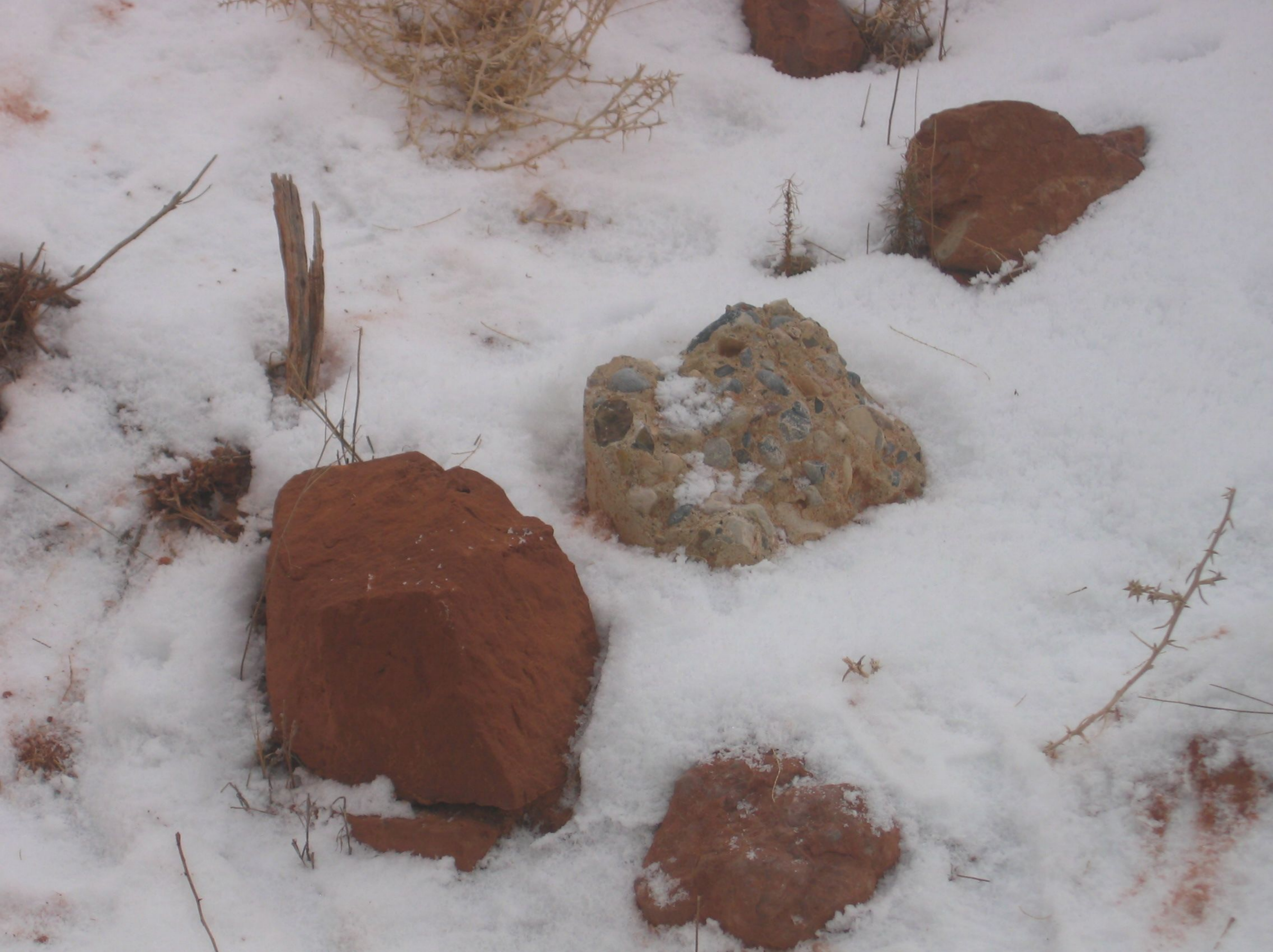
Hwy. Photo #30 - View of concrete cap found near the bottom of the 2:1 slope
