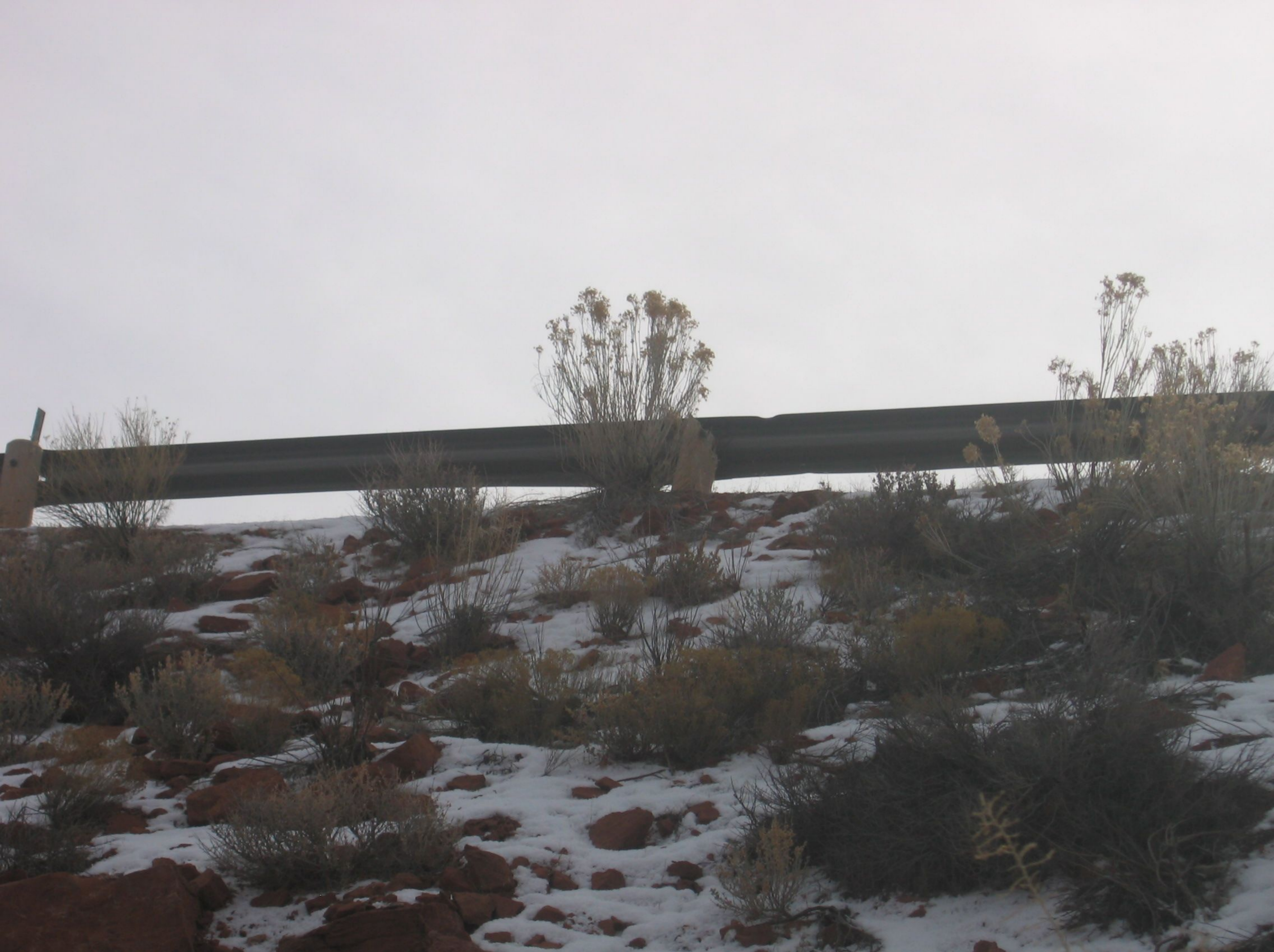
Hwy. Photo #29 - View of displaced concrete cap from guardrail support post in the area where the motorcoach contacted the rail.
