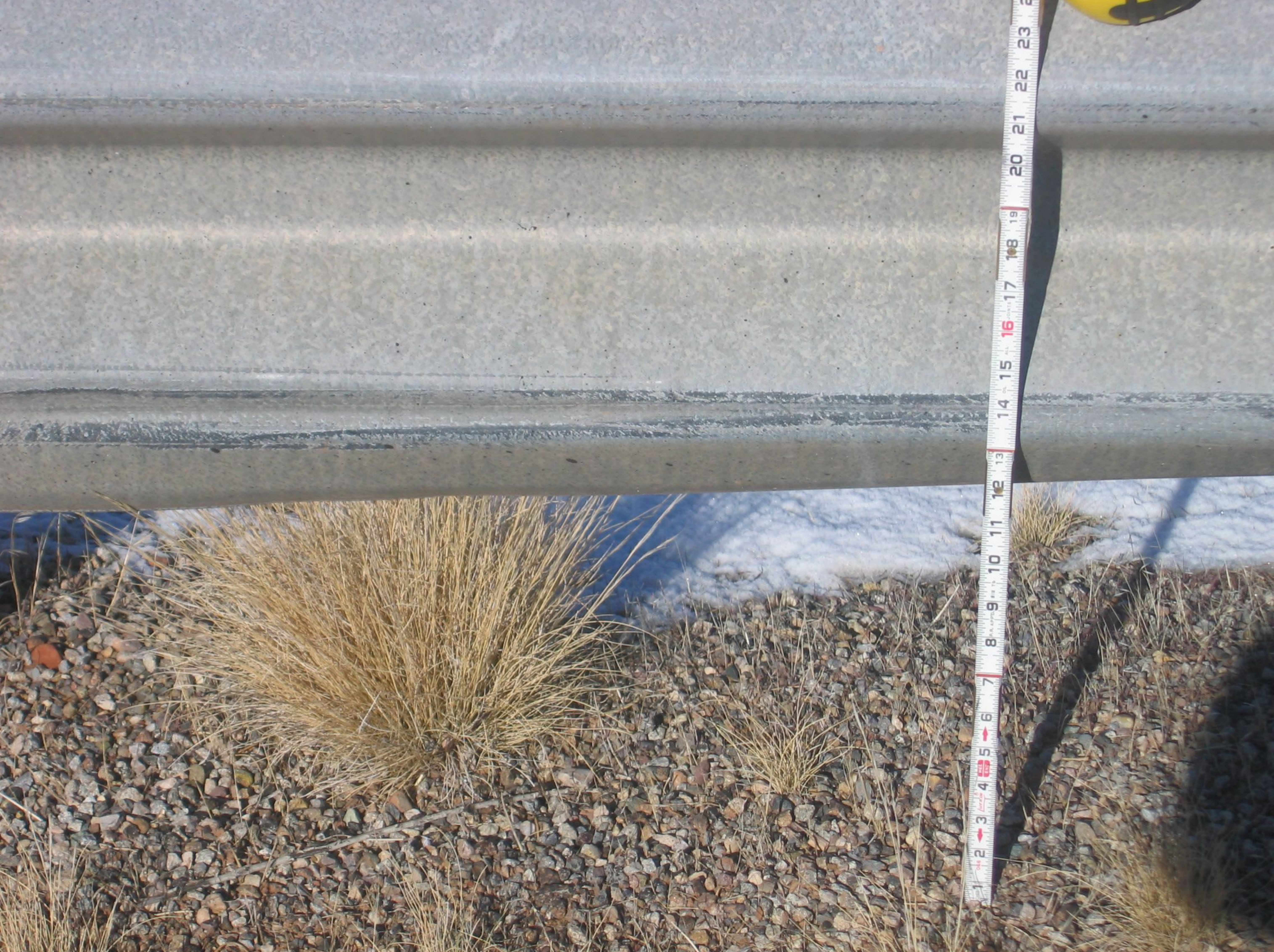
Hwy. Photo #24 - View of guardrail contact from motorcoaches lug nut covers
