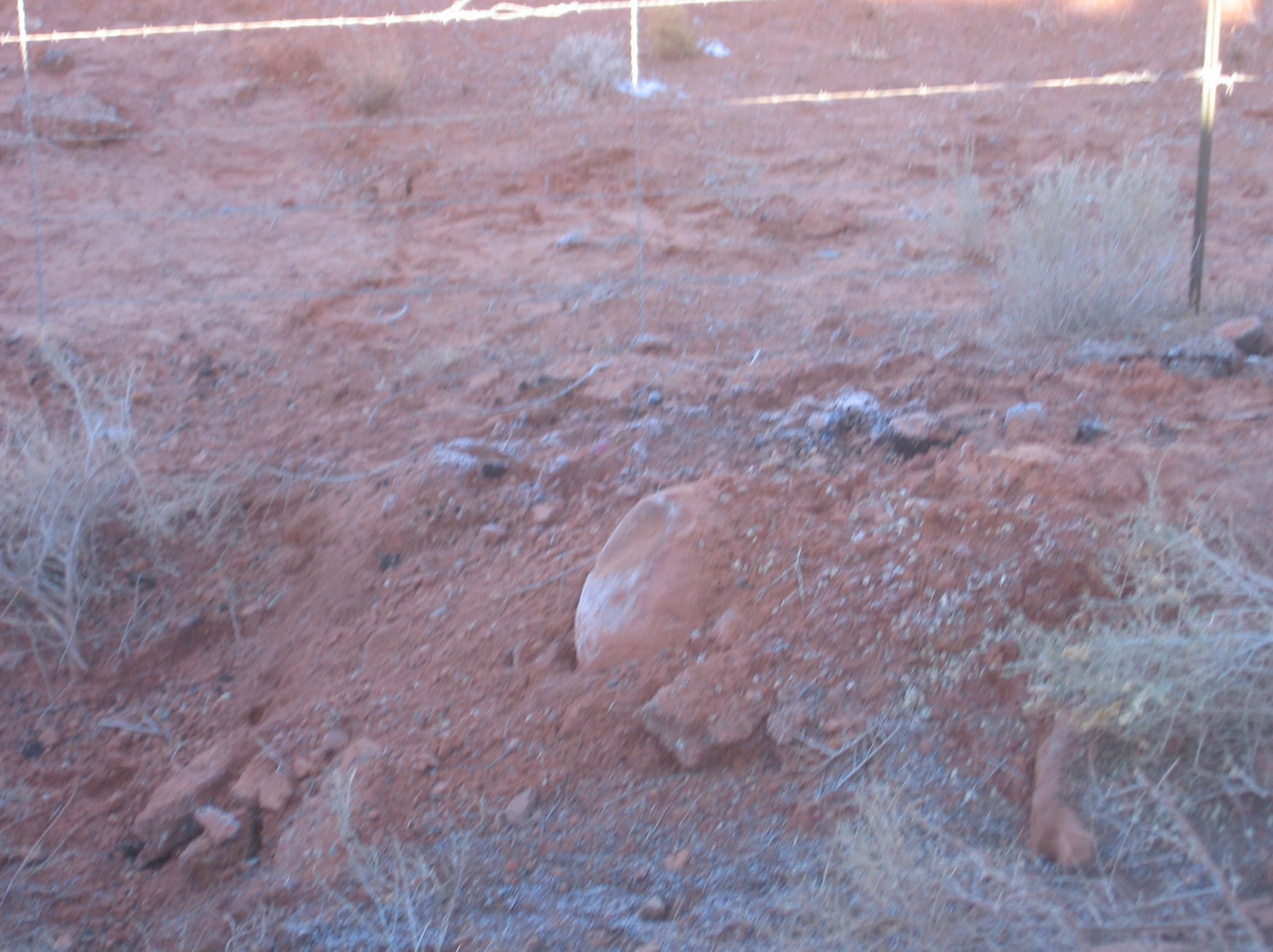
Hwy. Photo #19 - View of rocks in the area where the right rear and roof came down about 27 feet from the road edge.
