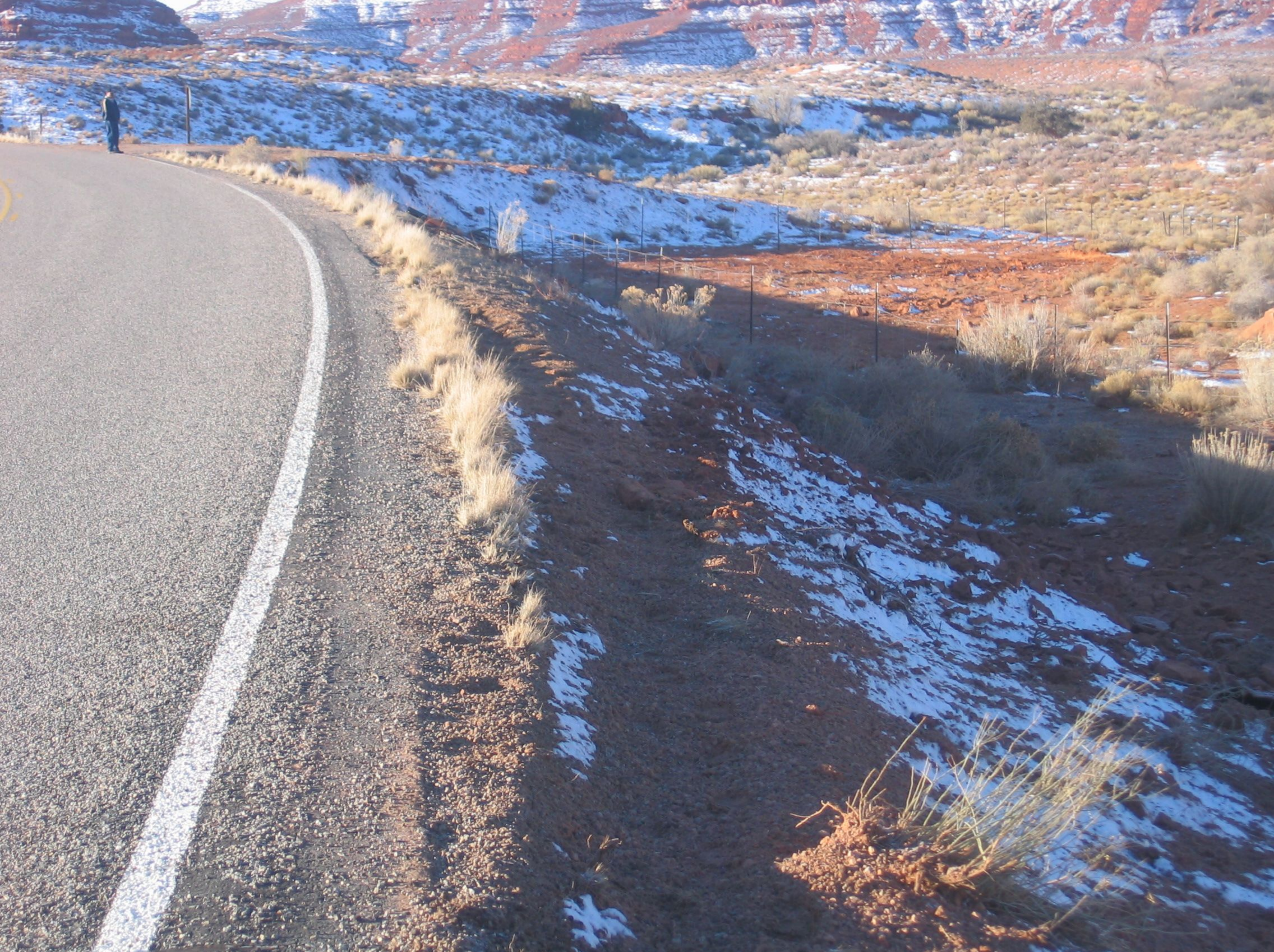
Hwy. Photo #16 - Note the steepness of the foreslope
