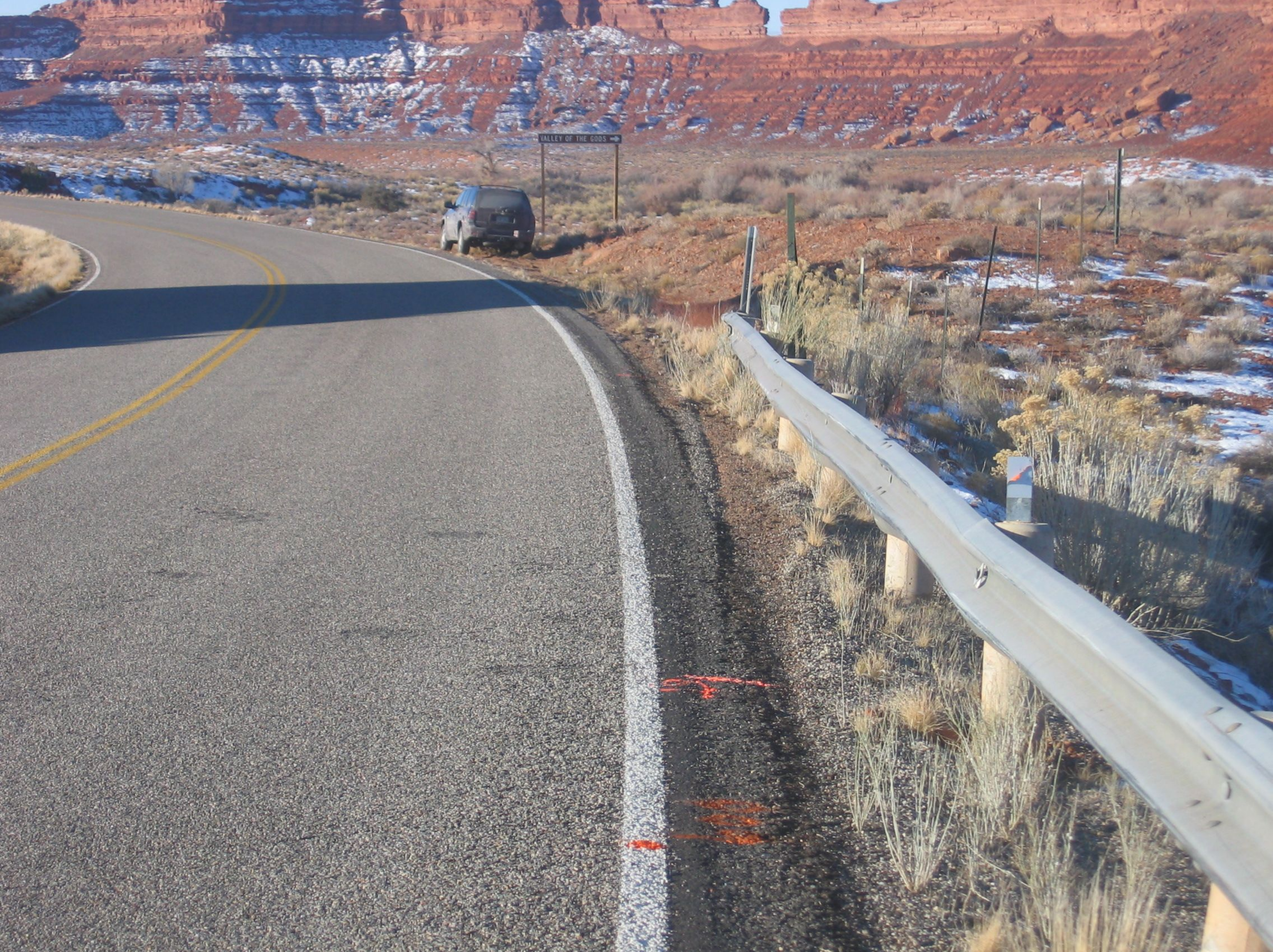
Hwy. Photo #11 - View of guardrail 61 feet from the end where the rear of the motorcoach came into contact with the rail.
