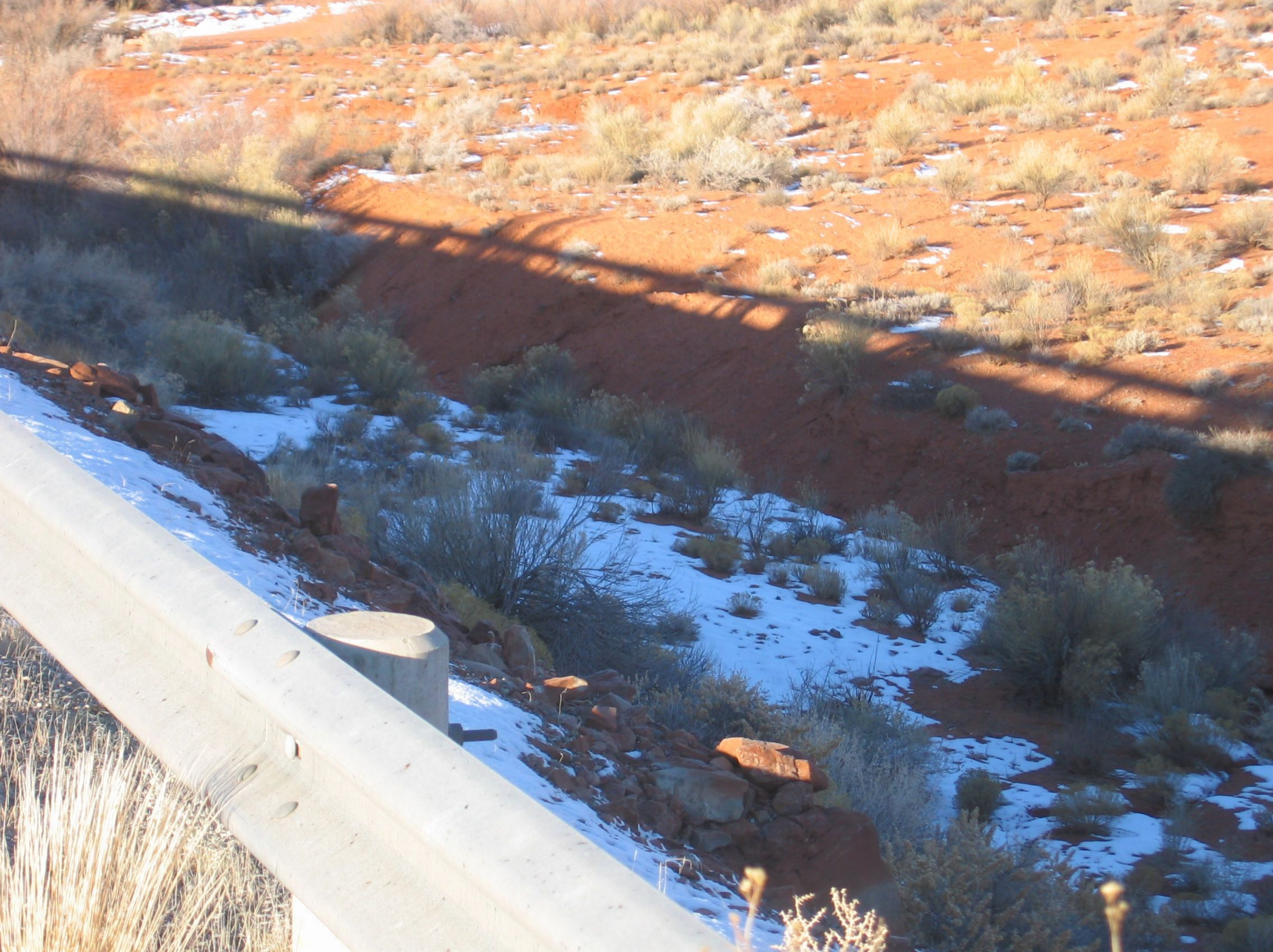
Hwy. Photo #8 - View of 2:1 slope on the backside of the guardrail with drainage culvert at the bottom of the slope.
