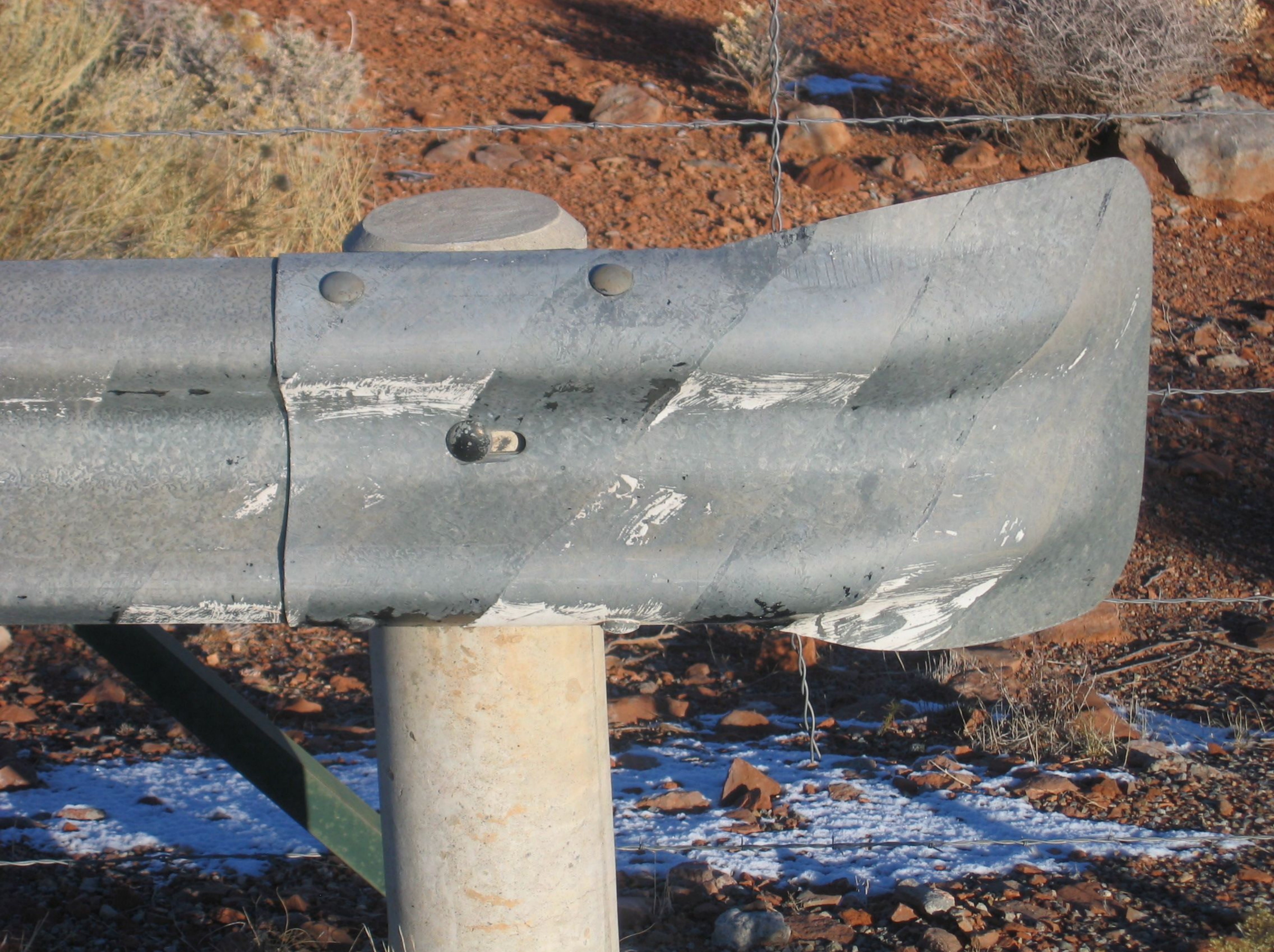
Hwy. Photo #7 - Close-up vie of guardrail end without safety end-treatment
