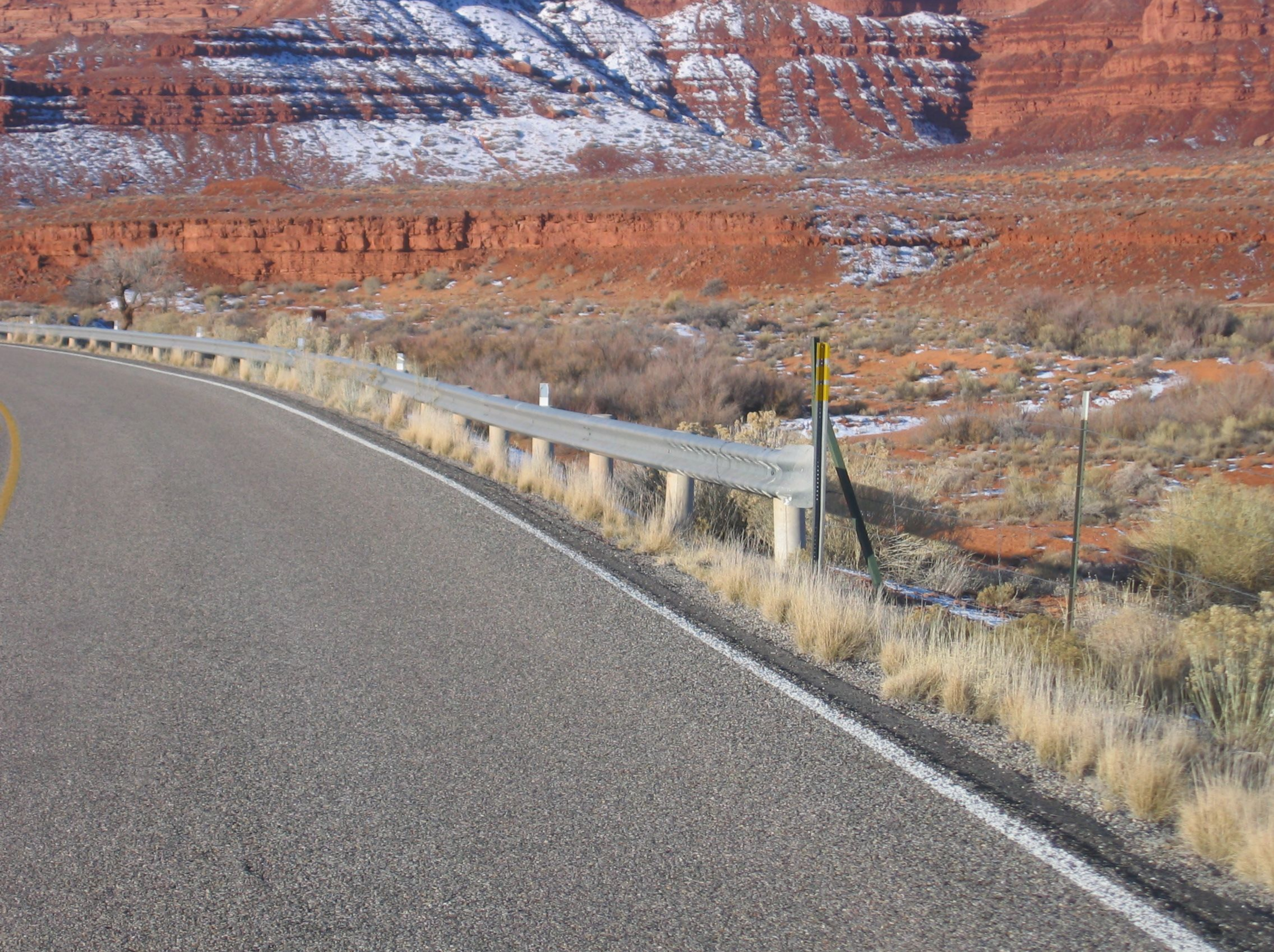
Hwy. Photo #6 - View of guardrail beginning 220 feet into the curve
