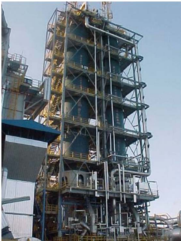
H-Oil Reactors in Poland
