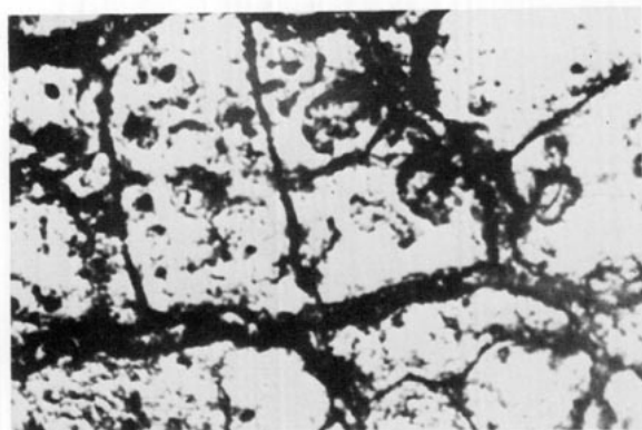
FIGURE 1. Small tears on the inside of PVC tubing after use in milking for about 1 year (1).
