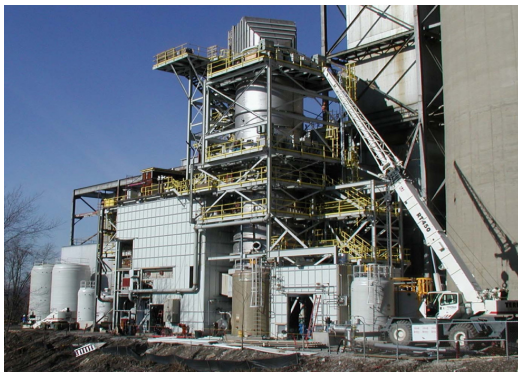
Powerspan's demonstration plant in Shadyside, OH, already cleans coal combustion flue gas to remove mercury vapor, \text{SO}_2 , and \text{NO}_x .
