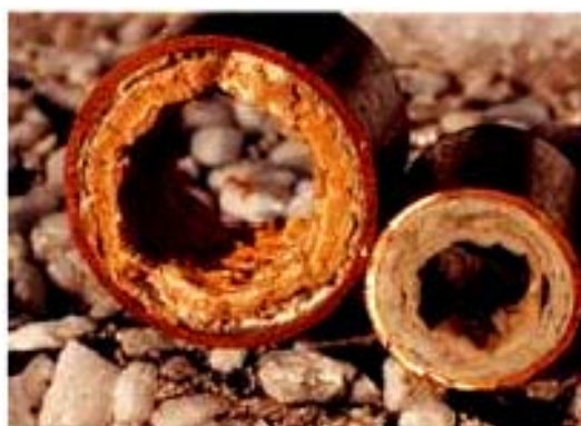
Figure 6. Example of Pipe Scaling
