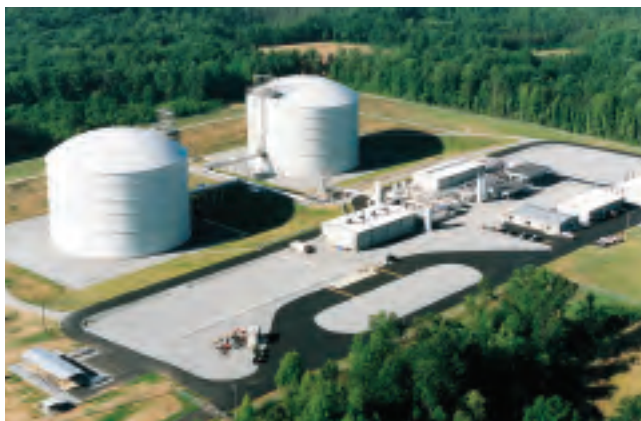
The Pine Needle, North Carolina peak-shaving facility, one of the largest in the nation, has a storage capacity of 4 Bcf. A sendout capacity of .4 Bcfd empties the tanks in 10 days of peak usage.
