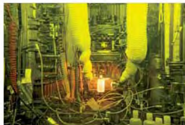
Hot cells at ORNL's Radiochemical Development Center are among the DOE hot cell facilities that may be used to test fuel recycle separations.
