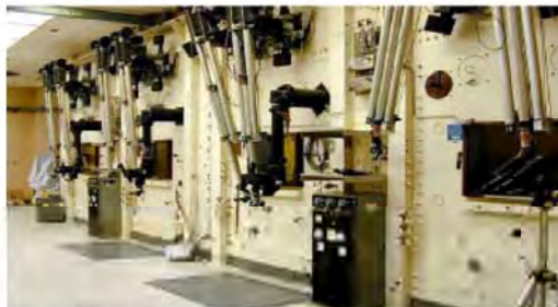
The Los Alamos Chemistry and Metallurgical Research Facility Wing 9 hot cells are used for irradiated fuel and materials examination, metallurgical examination, and neutron radiography.
