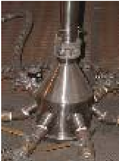
A "spider" is a mechanical device that splits activated carbon for mercury control from a single tube to multiple tubes and directs the carbon into injection lances before entering the flue gas duct.
