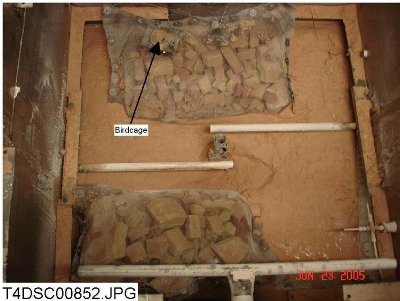
Figure 3-123. Birdcage and cal-sil baskets after the tank was drained.
