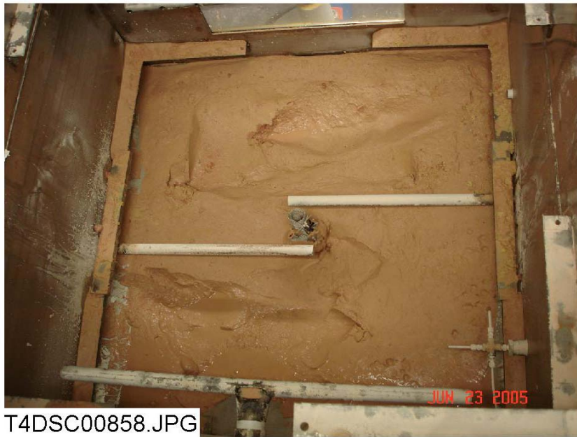
Figure 3-120. Sediment on the tank bottom.
