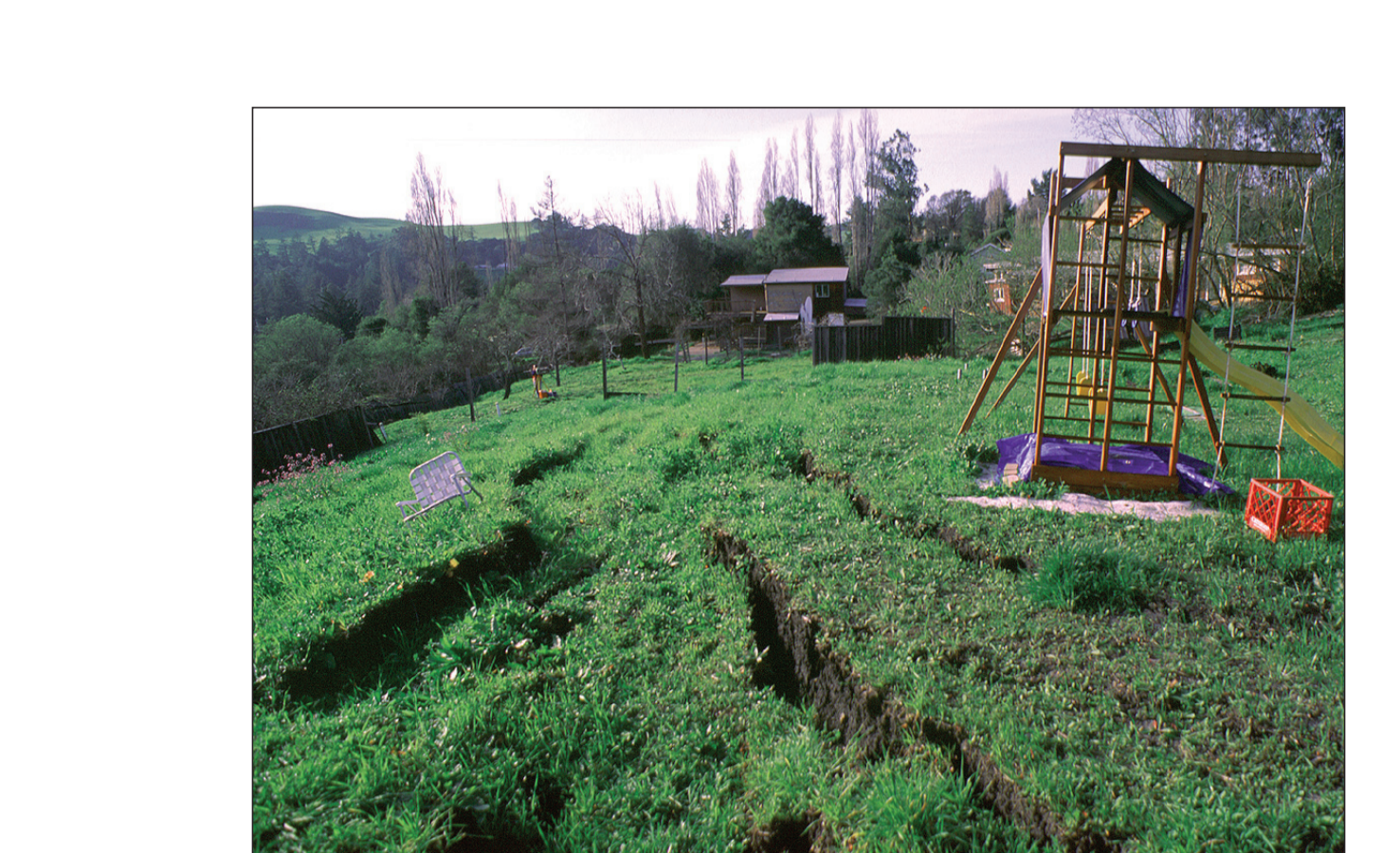
Figure 10. Graben that formed along axis of 'Lower ridge' of Scenic Drive landslide. View to west, photograph 21 March 1998.
