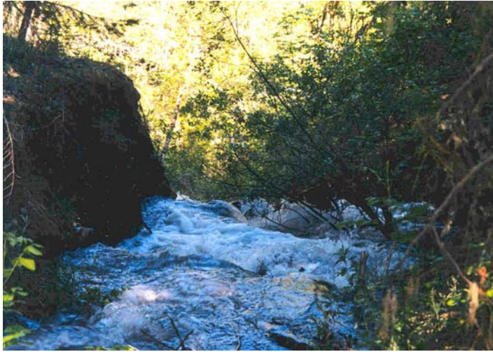
Figure 2-1. Near vertical wasteway banks
