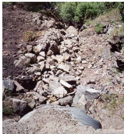
Figure 2-10. Example of backfill and riprap armament with minimal concrete and metal components
