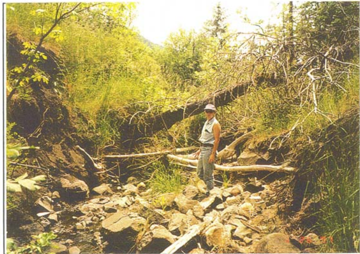
Photograph No. 1. Tyler Creek Wasteway. Looking downstream (southwest) near Station 47+33. Angular volcanic rock mostly 8 to 18 inches in size mantles channel bottom. Lateral cutting of banks is in progress. Note undercut tree toppled into channel. USBR Photograph by B.H. Carter, 6/26/97.
