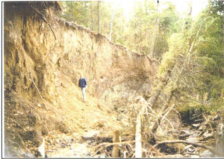
Photograph No. 10 Tyler Creek Wasteway. Looking downstream of Station 62+26, November 1993. Channel bank about 50 feet high in near vertical exposure. Panoramic Photograph No. 7, taken in 1997, shows this area failed back in flatter slope by landslide movement. USBR Photograph by B.H. Carter, 11/16/93.
