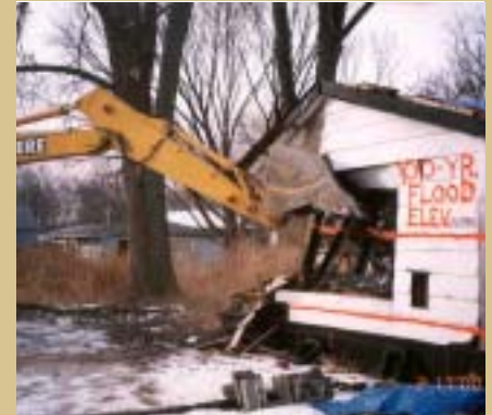
Buildings subject to deeper, fast moving, or repetitive flooding are prime candidates for acquisition. Older buildings are usually demolished.
