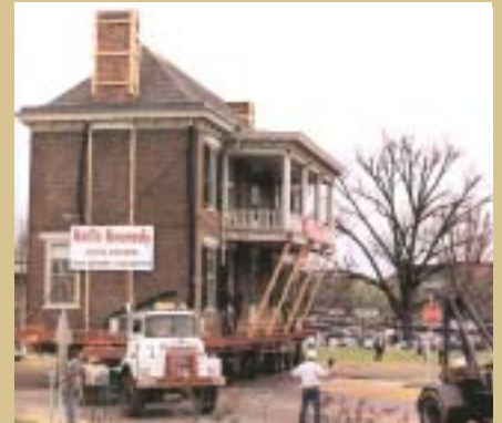
Moving this local landmark shows that nearly any building, no matter how big, can be relocated.
