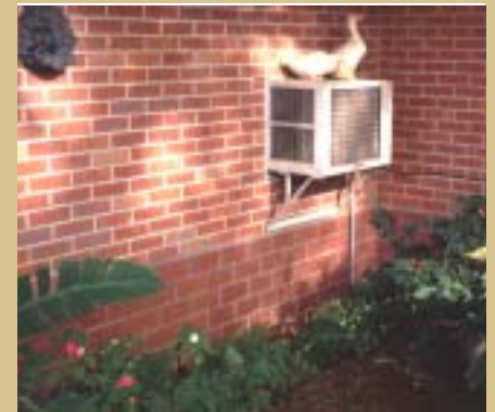
In this dry floodproofed Louisiana house, plastic sheeting is covered by thin facing brick. The building's walls become a watertight barrier to shallow flood waters.
