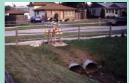
A series of culverts in Orland Hills, Illinois, obstructed flood flows, causing local flooding and necessitating repairs after every heavy rain. The Village used FEMA disaster assistance funds and State Motor Fuel Tax funds to enlarge and improve the culverts over several years. This systematic approach saved local funds and reduced flooding.
