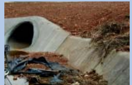
Runoff from bare ground causes erosion and fills in drainageways.
