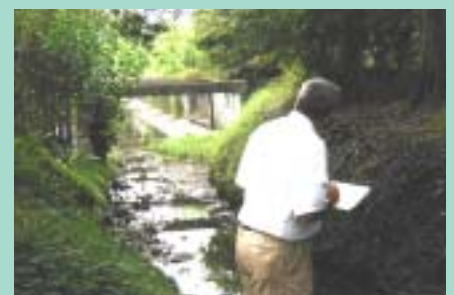
Jefferson Parish, Louisiana, has effective formal drainage inspection and maintenance procedures built on its NPDES program.
