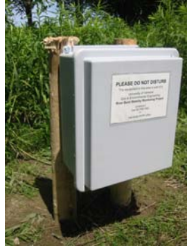
(a) Weatherproof box
