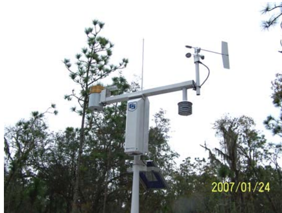
Figure 5. Campbell Scientific weather station installed in the study area.
