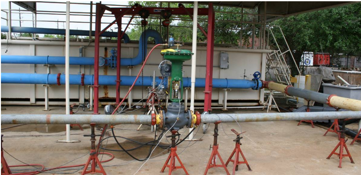
a) The 4-inch Fisher ES valve installed at KEI
