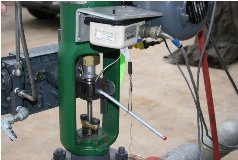
b) The Crane ForceLink used to measure thrust and LVDT used to measure stem travel
