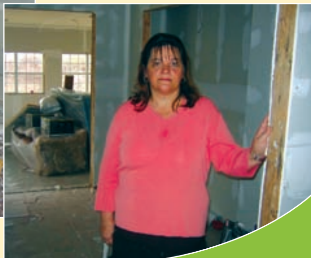
Homeowner Claudette Luther stands within the hollowed-out walls of her home under repair with SBA disaster funds
