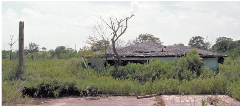
An abandoned house in the Brownwood subdivision
