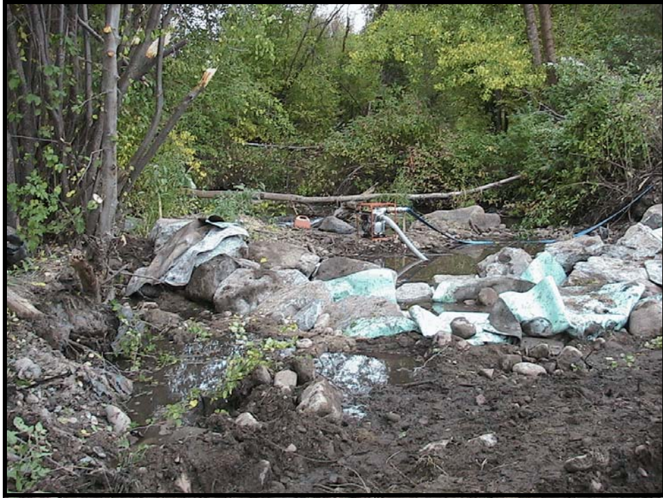
Photo A-7. Downstream view of Weir No. 1; the non-permeable geomembrane has been installed but not fully covered.
