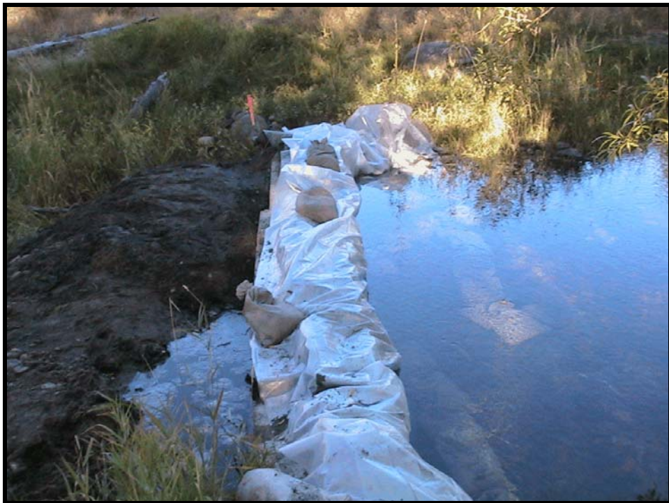
Photo A-2. The ecology block and plastic cofferdam was set about 80 feet upstream from the original diversion dam.
