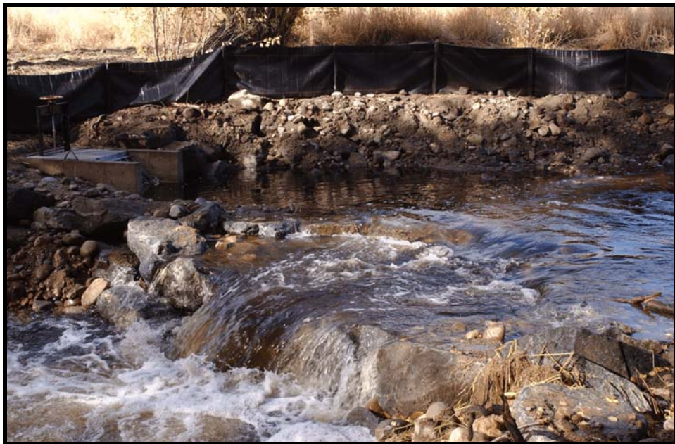
Photo A-24. November high flow over the double-drop Weir No. 1, which is the diversion control structure.
