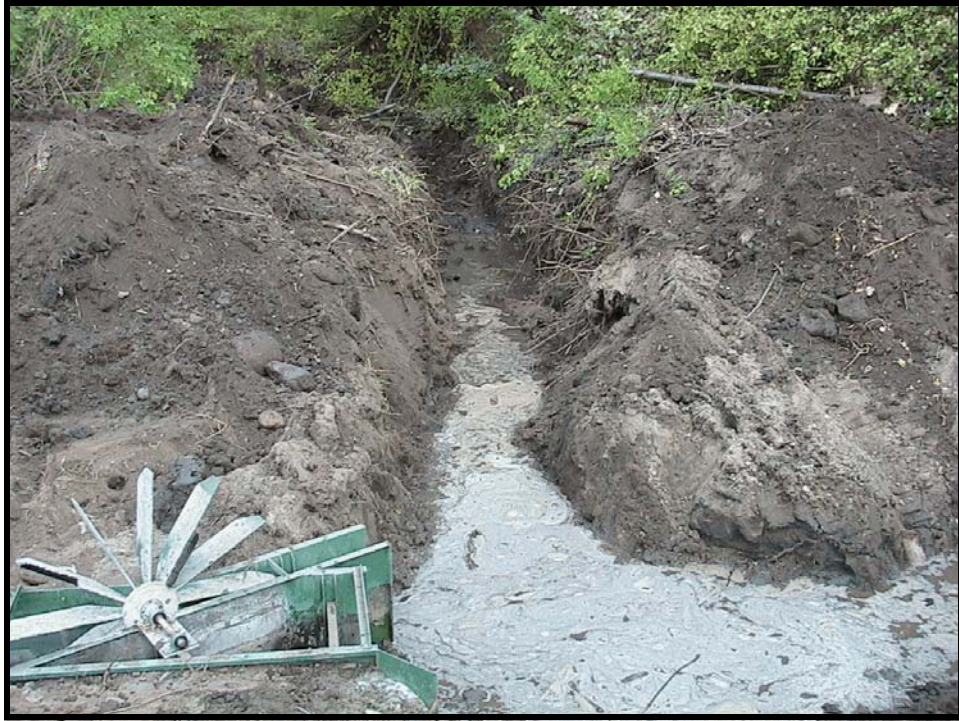
Photo A-15. The fish bypass channel, before installation of the fish bypass return pipe.
