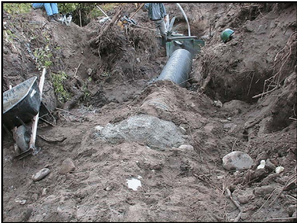
Photo A-12. The concrete protects and weights the transition between the PVC (white) and HDPE (black) irrigation pipes (see photo A-10). The fish screen is in the upper center of the photo, just above the black pipe.
