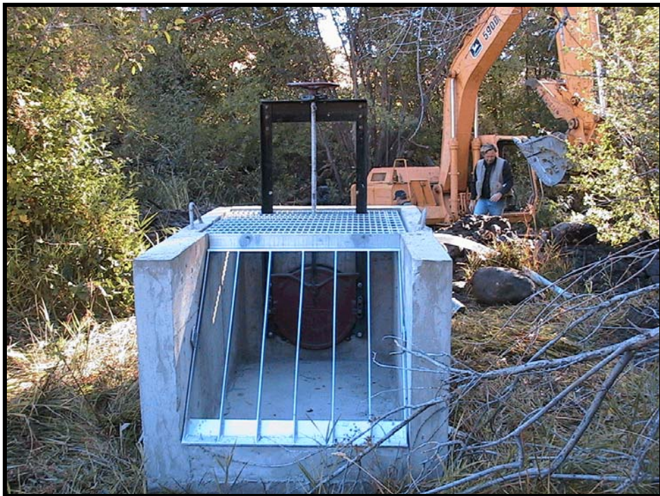
Photo A-8. The intake side of the new diversion box, before placement. Both the trashrack and the grate(on top) are galvanized.
