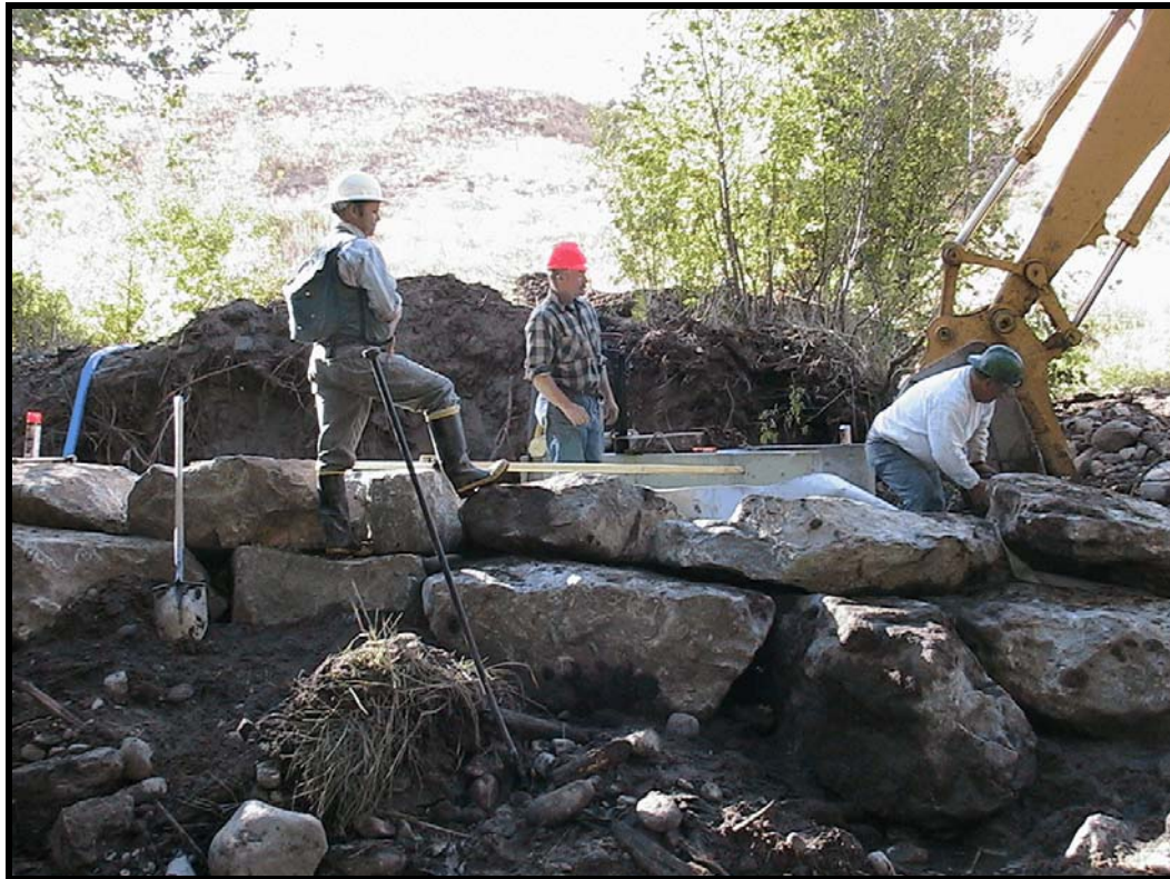
Photo A-5. Looking upstream at the left arm of Weir No. 1. Diversion structure is set in the center of the photo. The large rocks were brought in from a quarry about 30 miles east. Note the even slope of the rocks and lack of gaps between them.
