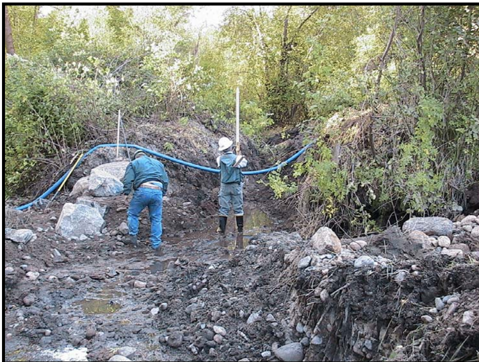
Photo A-4. Looking downstream at site of Weir No. 1 as technicians set elevation for the new diversion structure. The existing ditch was excavated about 12 inches to serve the lower elevation of the new headgate.
