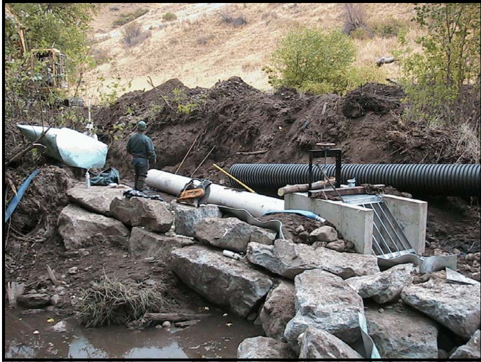
Photo A-10. Looking upstream across the right arm of Weir No. 1. The white PVC pipe is attached to the box's "stub." In a field modification to extend the irrigation further down the ditch, the corrugated black HDPE pipe was attached to the PVC pipe.
