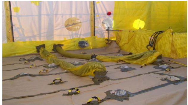
Exhibit 4-18: Secondary portable HEPA exhausters.
