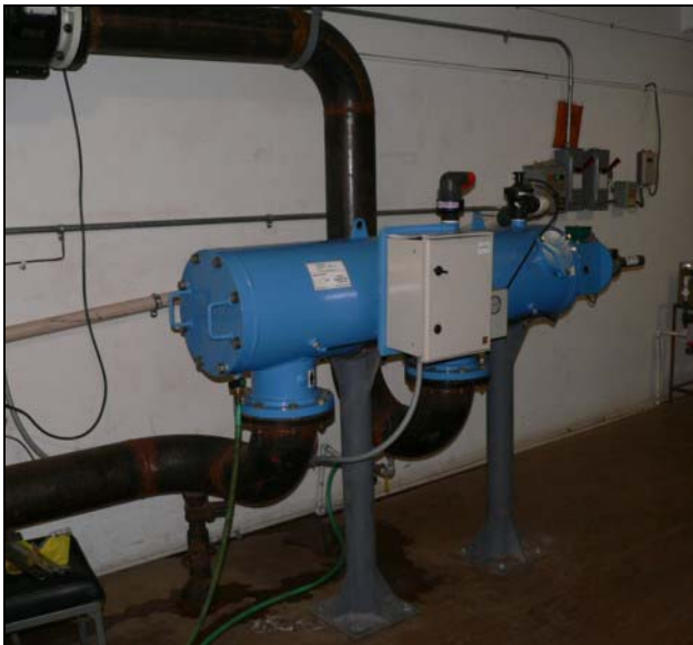
Figure 1. – 450 GPM filter installed at Parker dam.
