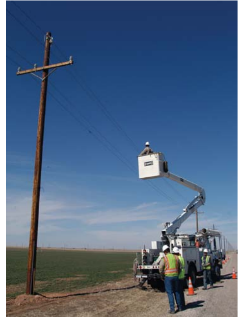
INFRASTRUCTURE UPGRADES: As part of the new electrical distribution system at the Pantex Plant, approximately 19 miles of overhead line will be replaced.
