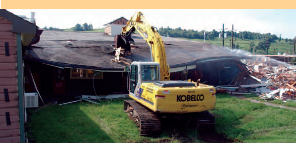
MILESTONE MACHINE: A track hoe knocks down a portion of the roof of the former technical library at Y-12, one of 258 structures demolished so far.
