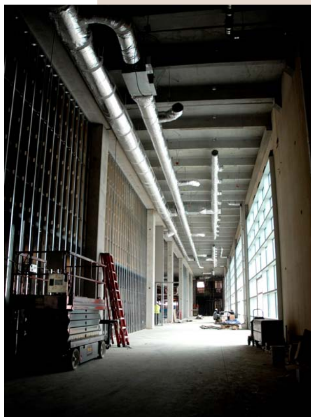
JACK CASE CENTER: This corridor filled with natural light from large windows leads to the new cafeteria that will be located in the Jack Case Center.
