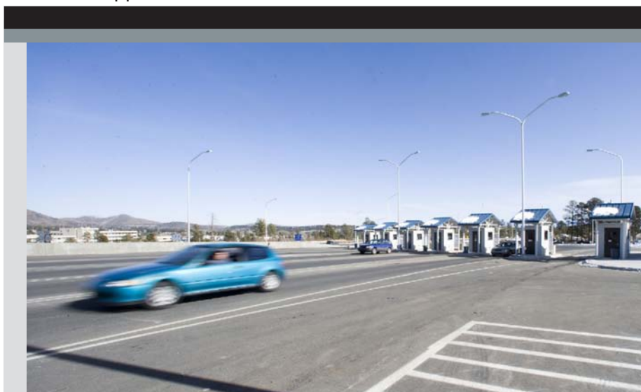
PERIMETER SECURITY: New vehicle access portals have been constructed and are now operational for all westbound vehicles coming into the Los Alamos National Laboratory Technical Area 3, or traveling to the Pajarito Ski Hill, and other areas on West Jemez Road near the New Mexico laboratory.
