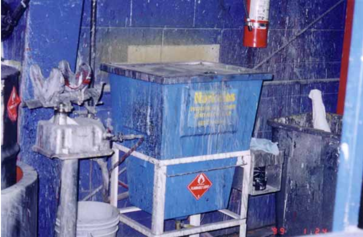
Figure 3-5. Spray Gun Cleaning System at Holmes.
