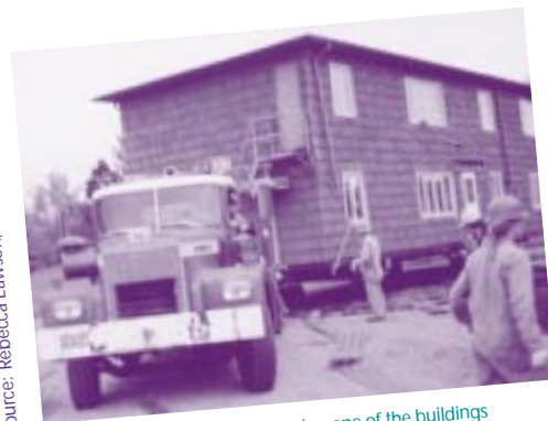
Contractor moving one of the buildings for the Bagley Downs apartment complex
