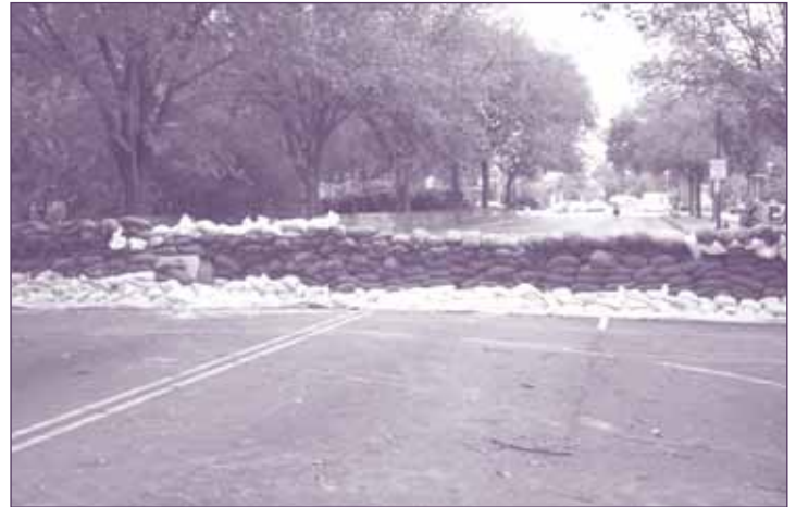
Temporary sandbag and jersey barrier closure at 17th Street constructed by the National Park Service in preparation for Hurricane Isabel
