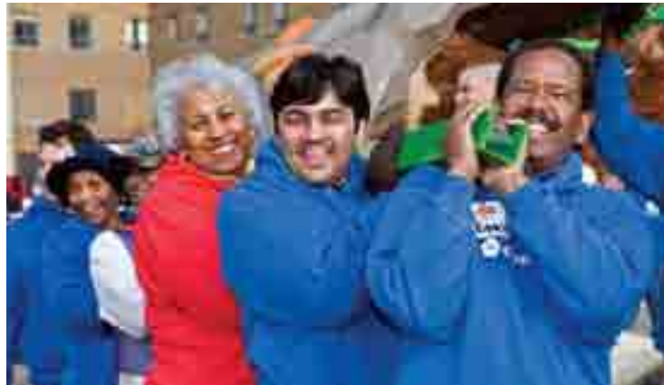
THIS PAGE: In Highland Park, Michigan, volunteers build a playground for children in a low-income neighborhood.
