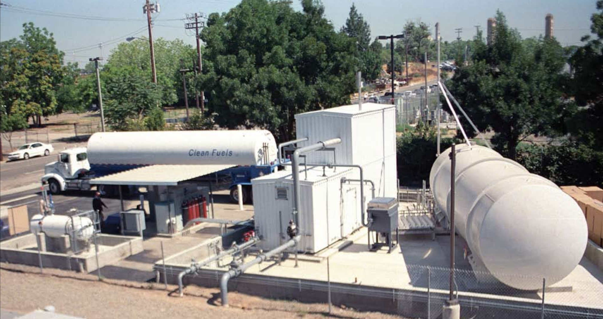
Compact High Efficiency Natural Gas Liquefier located at 2001 Front Street in Sacramento, Calif.
