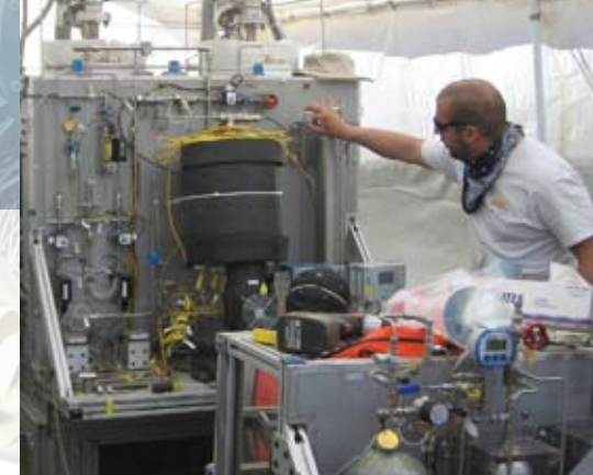
Checking the condenser subsystem on the NASA oxygen production system
