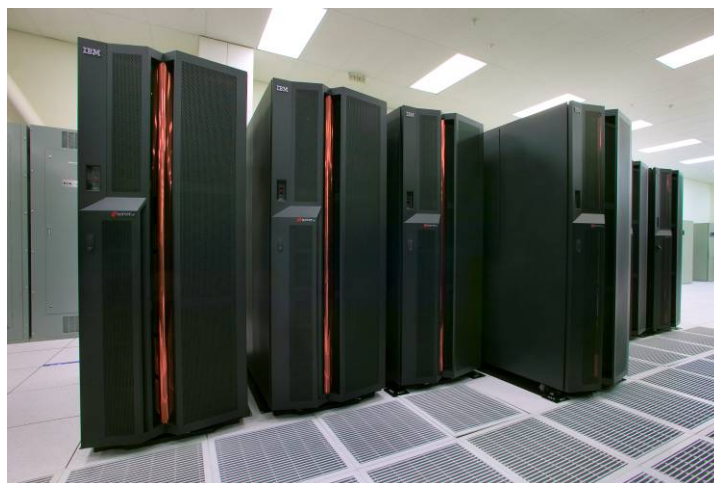
Figure 12. Bassi is an 888-processor IBM p575 POWER5 system with a theoretical peak performance of 6.7 teraflop/s.
