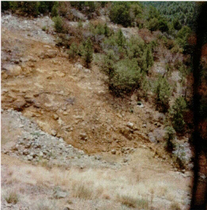
Photo 4: Dry (vegetated) drainage of Little Walnut Creek from the former West tailings area, July 17, 2002
