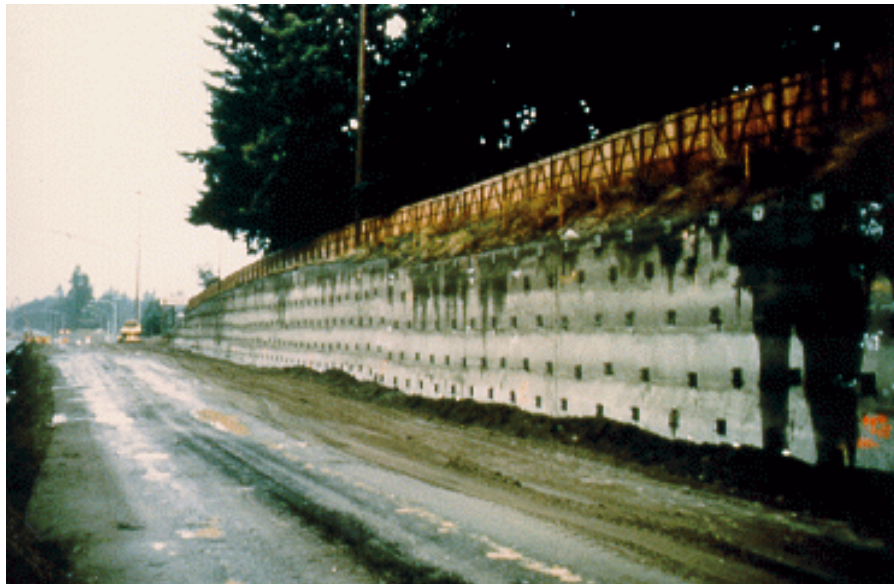
Figure A-2. Black Lake Interchange, WSDOT Olympia, WA - Soil Nail Wall Construction
