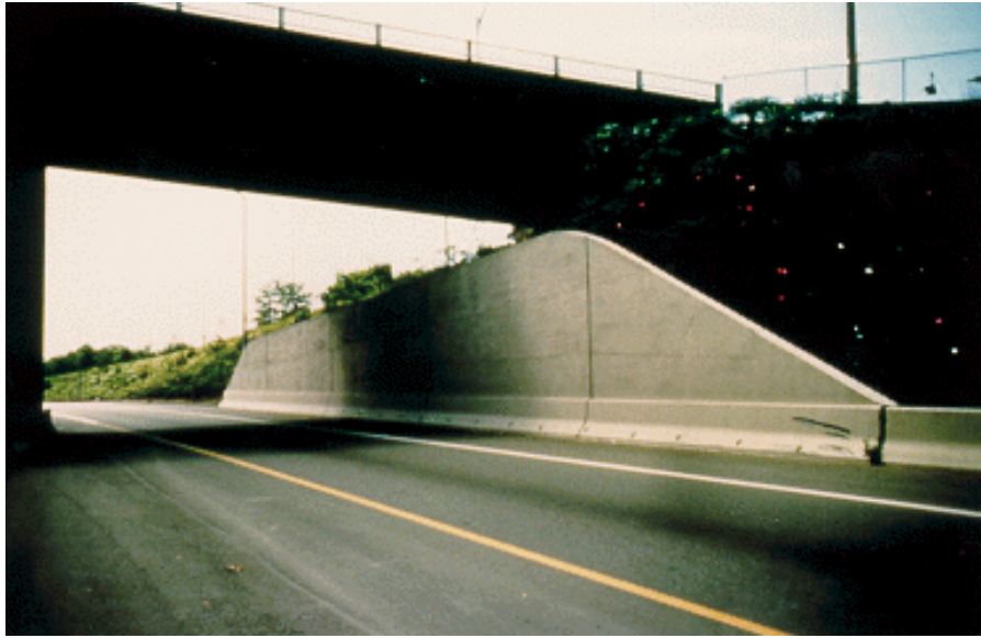
Figure A-5. I-5, WSDOT Tacoma, WA - Soil Nail Wall in Tacoma (Bridge End Slope Removal)
